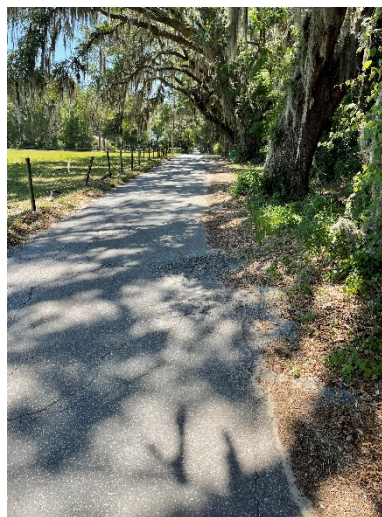
Photo 1: Tree roots under the asphalt pavement
